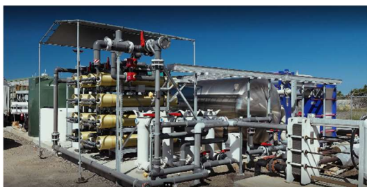
The demonstration project was conducted at Trevi Systems' desalination plant.
